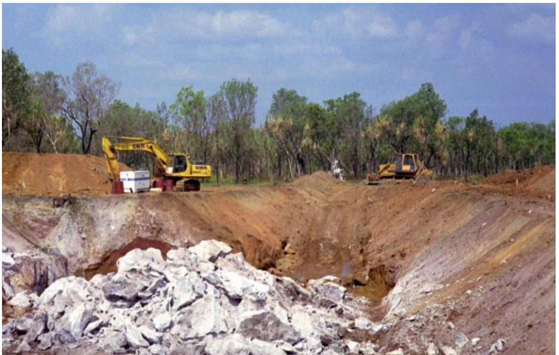
Figure 5 Test mining of magnesium at Winchester during the wet season (after blasting Level 0)
