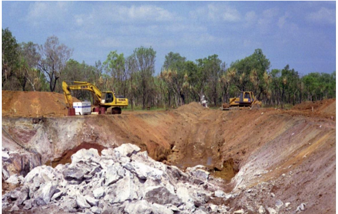
Figure 4 Test mining of magnesium at Winchester during the wet season (after blasting Level 0)
