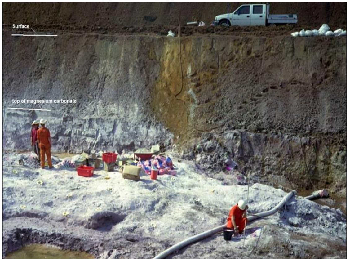
Figure 5 Test mining of magnesium at Winchester during the wet season (preparing to blast Level -1)
