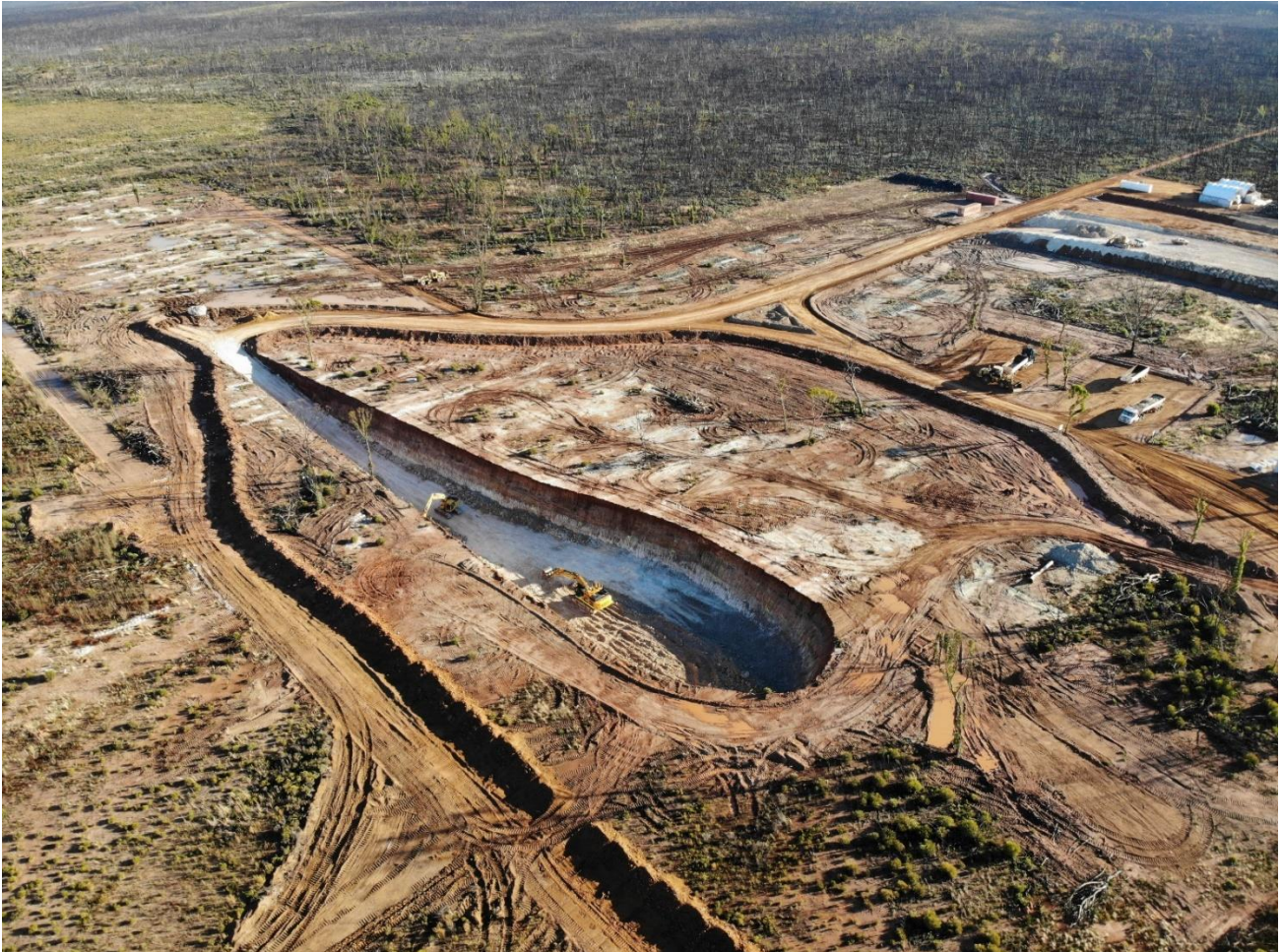
Figure 2: Aerial view of pit – Showing overburden almost removed prior to first ore exposure.
