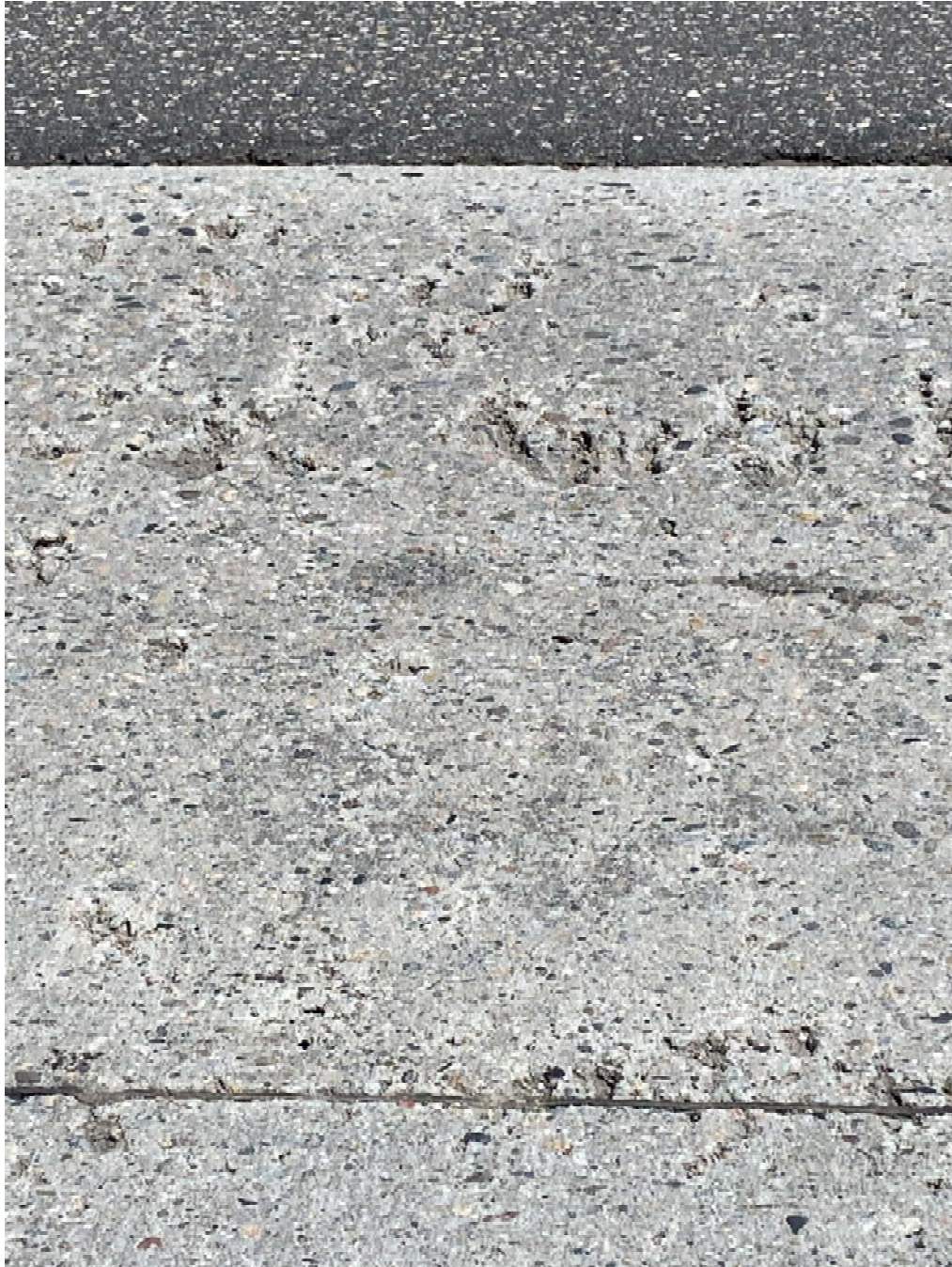
Figure 7 Mid-Section Reference Slab -12 months Close up Figure 3 Scaling, Surface Damage, Pitting and Aggregate Pop Outs
