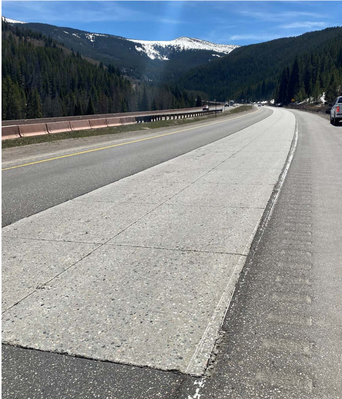
Figure 5 Beginning-Section Reference Slab -12 months Top concrete surface worn off, Cracking, Scaling, Surface Aggregate Pop Outs, Rutting, Joint Rot
