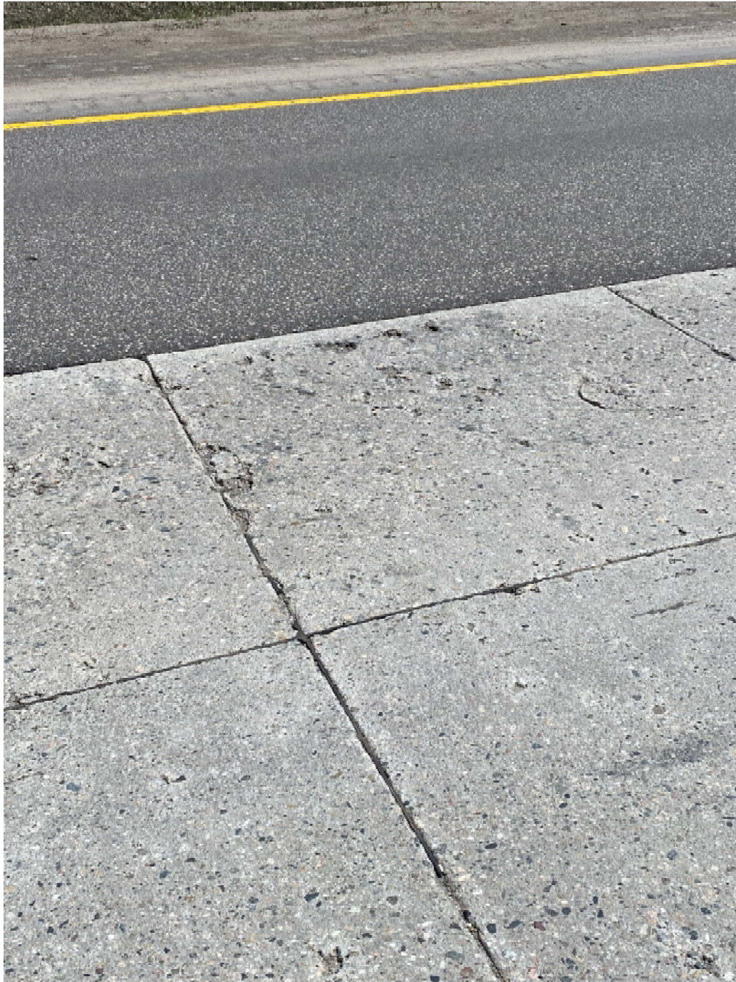
Figure 8 Mid-Section Reference Slab -12 months Close up Figure 3 Severe Surface Damage, and Joint Rot
