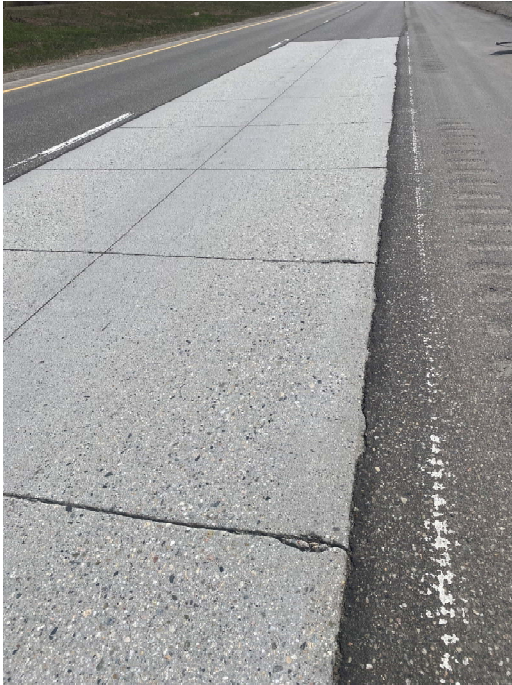
Figure 19 End-Section Silica Fume Slab - 12 months Top concrete surface partially worn off, Scaling, Pitting and Aggregate Pop Outs, Joint Rot
