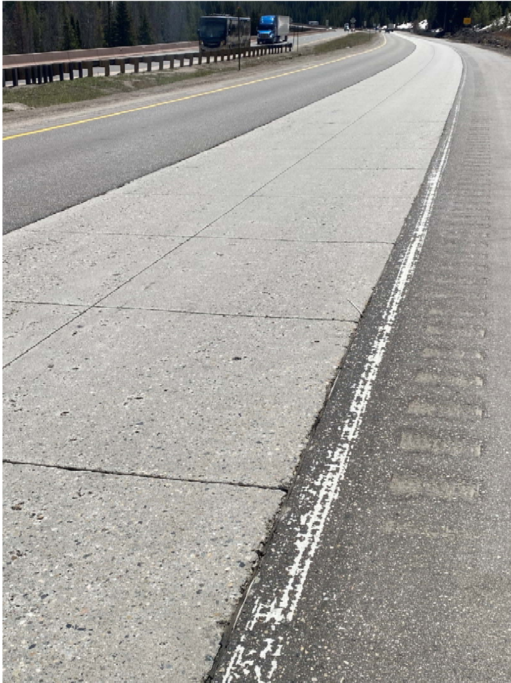
Figure 10 End-Section Reference Slab - 12 months Scaling, Surface Damage Aggregate Pop Outs
