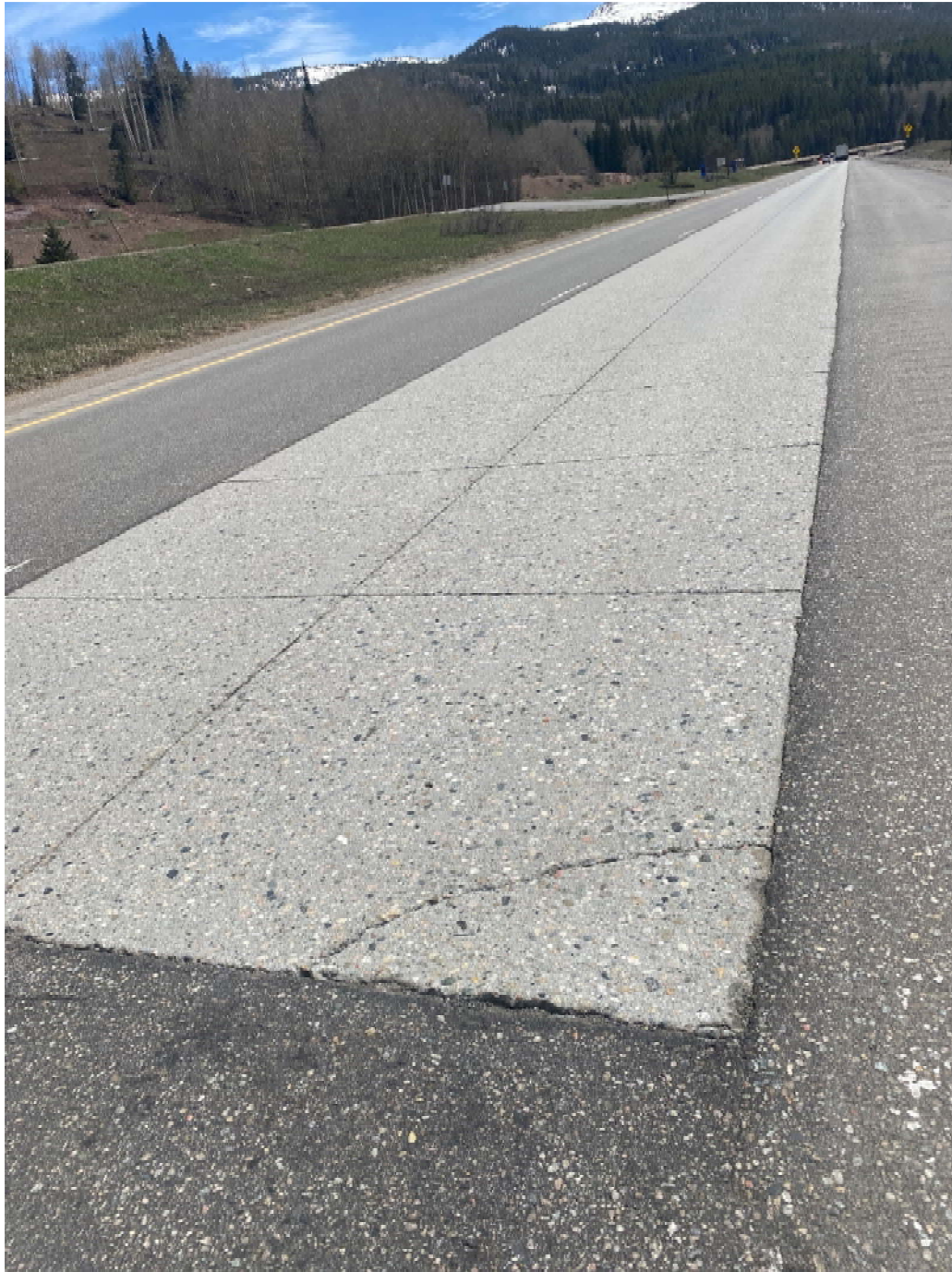
Figure 16 Beginning-Section Silica Fume Slab – 12 months Top concrete surface worn off, Scaling, Cracking, Pitting and Aggregate Pop Outs, Joint Rot
