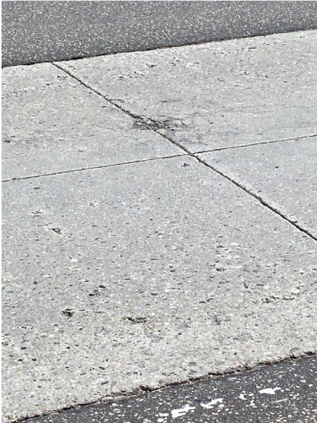
Figure 9 Mid-Section Reference Slab -12 months Scaling, Surface Damage, and Joint Rot
