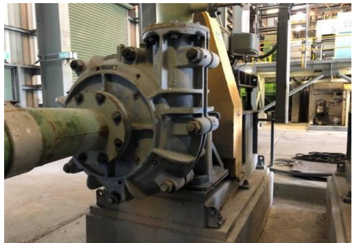
Grinding Section Asset 1B - 9 - 10/8 Pump
