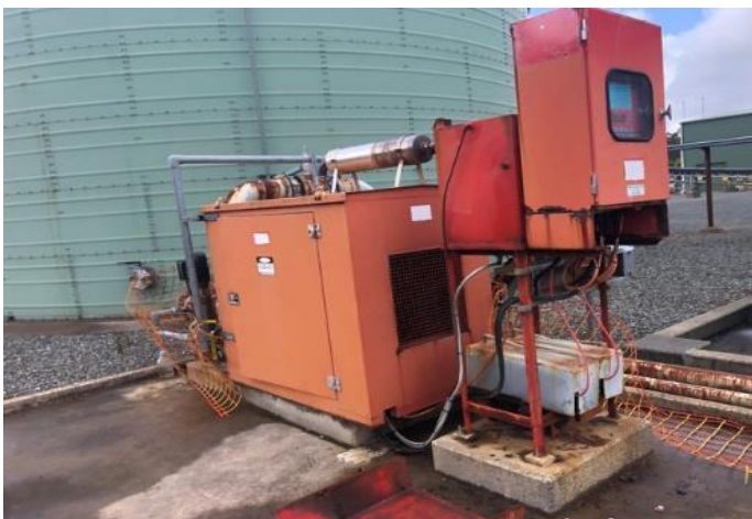
Water Section Asset 1H - 2 Fire Fighting Pump
