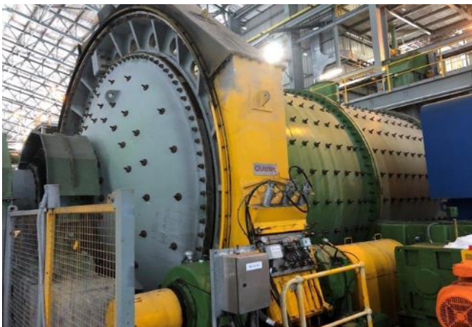
Grinding Section Asset 1B - 6 - Autotec Ball Mill
