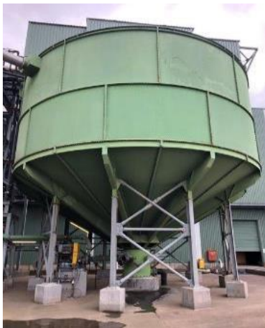
Thickener Section Asset 1E - 13 - Outotec High Cone Thickener
