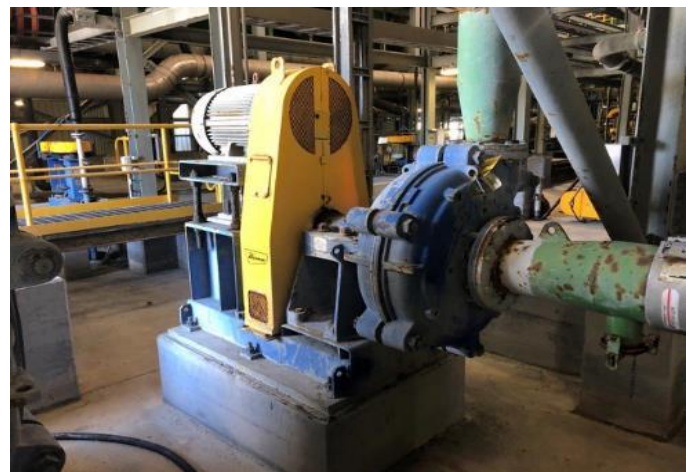
Regrind Section Asset 1D - 2 - 8/6 Pump
