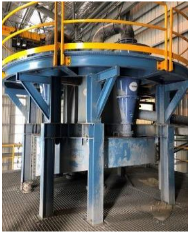
Grinding Section Asset 1B - 11 - Krebs Cyclones
