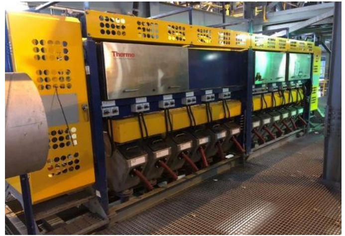
Tails Section Asset 1E - 4 - Multi Stream Analyzer
