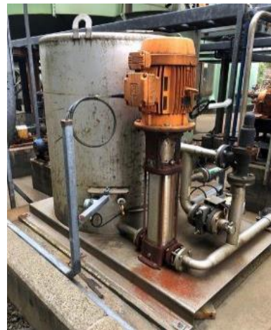
Concentrate Section Asset 1F - 6 - Pump & Tank
