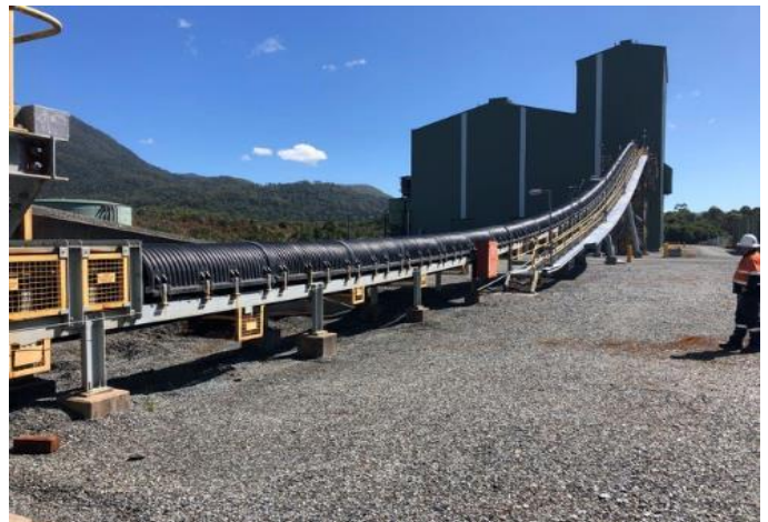
Grinding Section Asset 1B - 4 - Main Infeed Conveyor
