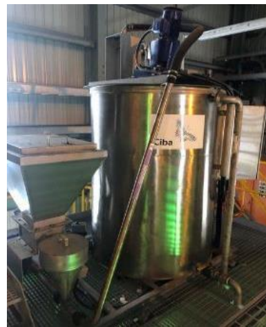
Reagents Section Asset 1G - 5 - Ciba Flocc Tank
