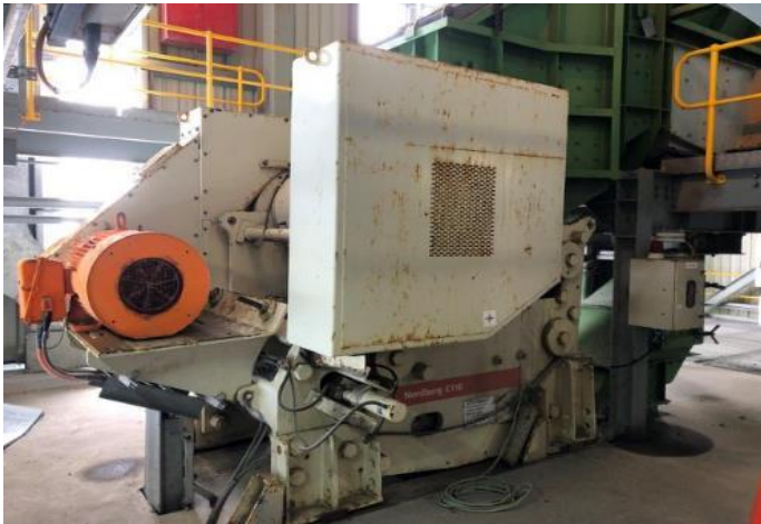
Crushing Section Asset 1A - 3 - Jaw Crusher
