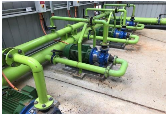
Water Section Asset 1H - 14 - Pumps
