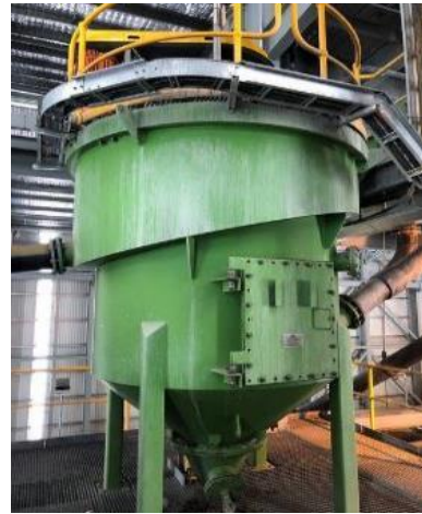
Grinding Section Asset 1B - 12 - Flash Flotation Cell
