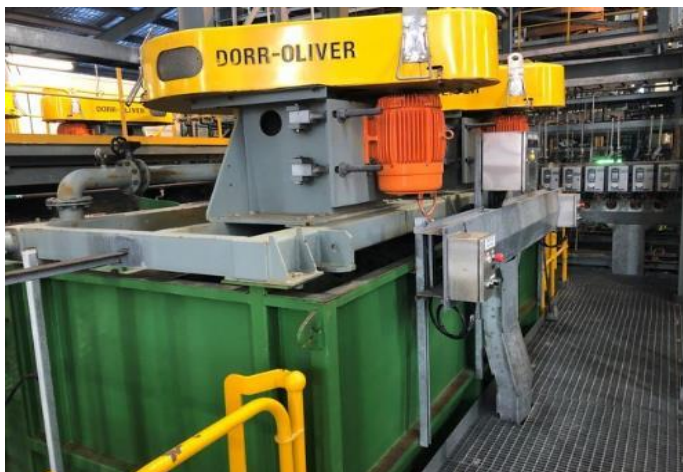
Flotation Section Asset 1C - 14 - Bank of 2 Flotation Cells
