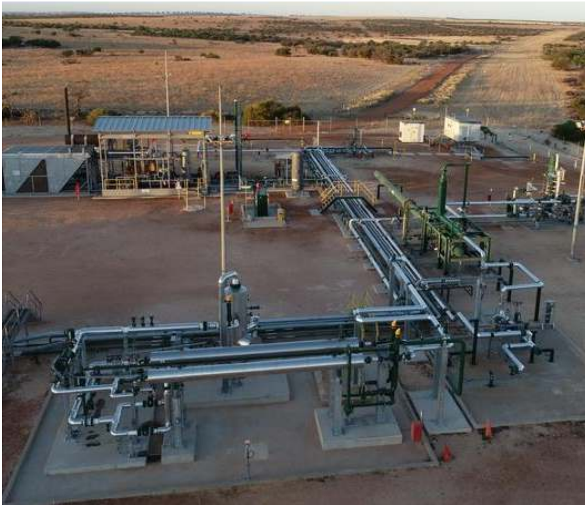
Image 3: A DBNGP connection point
