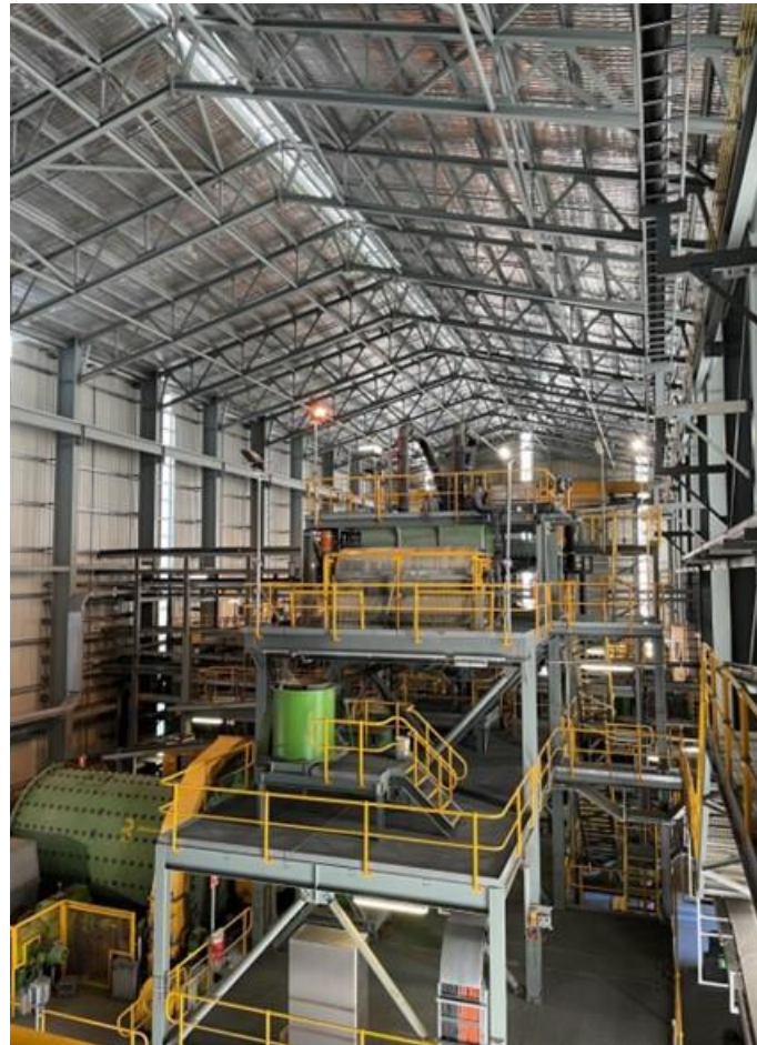
Grinding and Flotation Circuits
