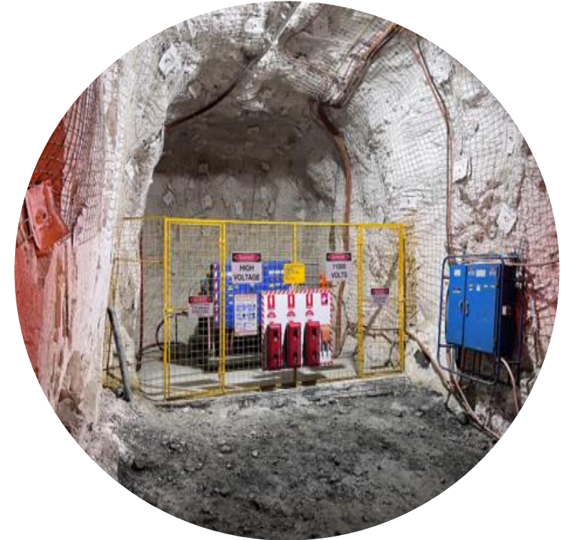
Underground Electrical Substation
