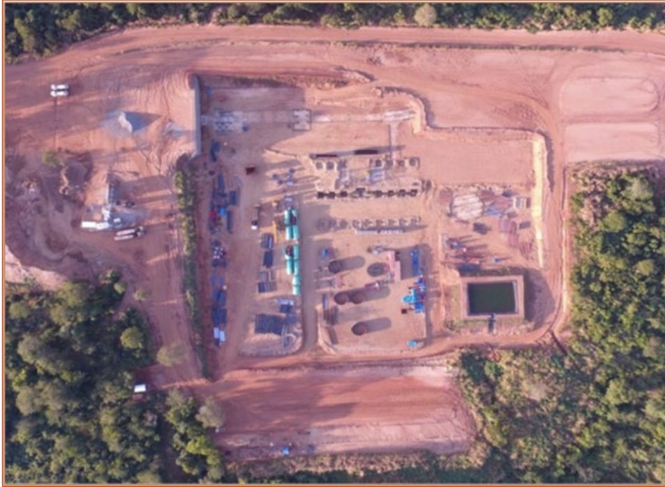
Figure 2: Top view of the processing plant area. Numerous pieces of equipment visible including the floatation cells, filter presses, crushers, screw classifiers, fine ore bin sections and laydown of the structural steel components.
