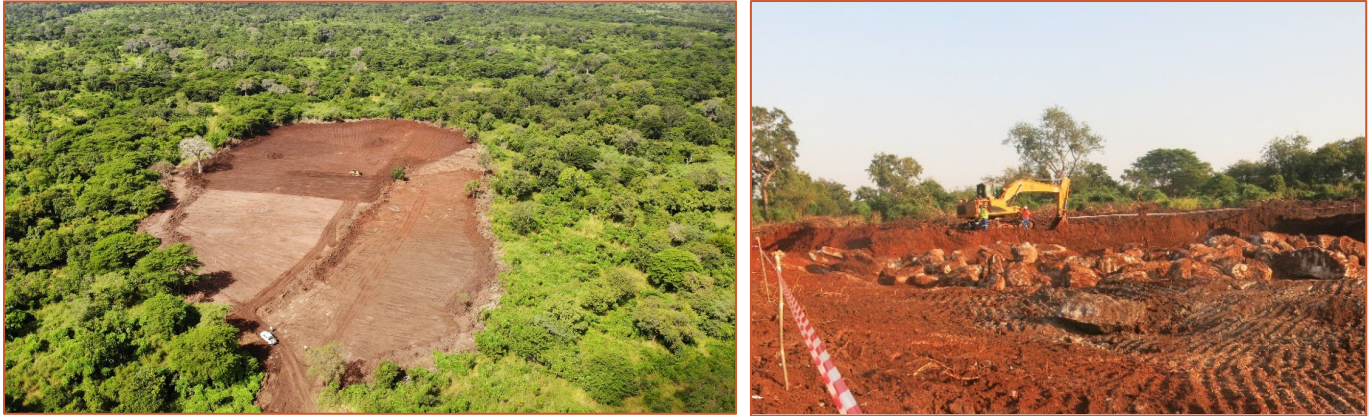
Figure 6: Starter pit pre-strip. The area is approximately 700m to the west of the Processing Plant area. Approximately 0.30 to 1m of clay rich saprolitic waste material has been used in the construction of the TSF.
