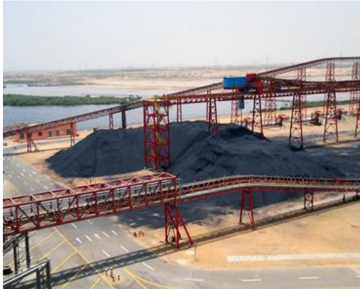
Figure 19: Typical mobile tripper stockpile elevated belt conveyors
