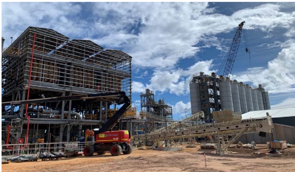
Figure 1 Lucky Bay Processing Plant
