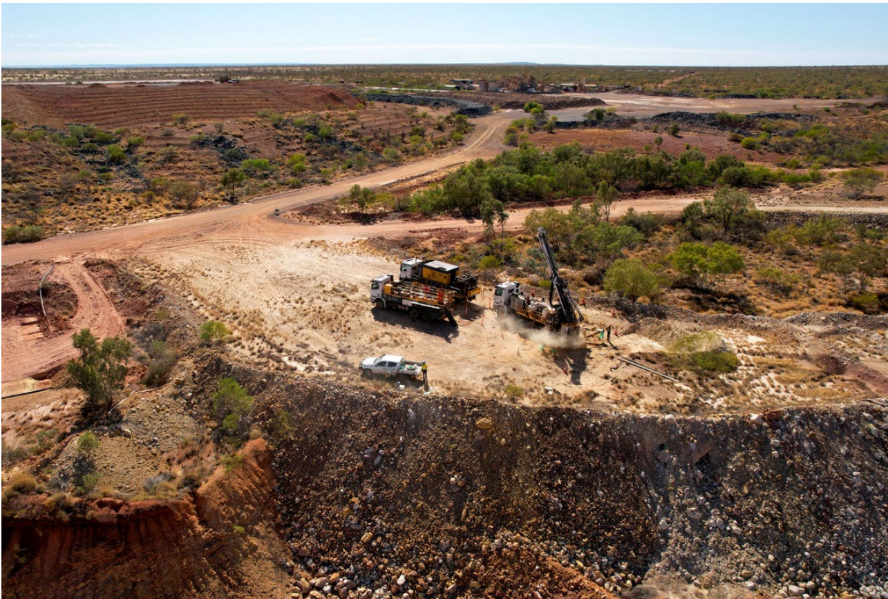
Figure 1: RC drilling for the extension and upgrade of the Speedy open pit Resource with ROM stockpiles, processing facility and camp in the background
