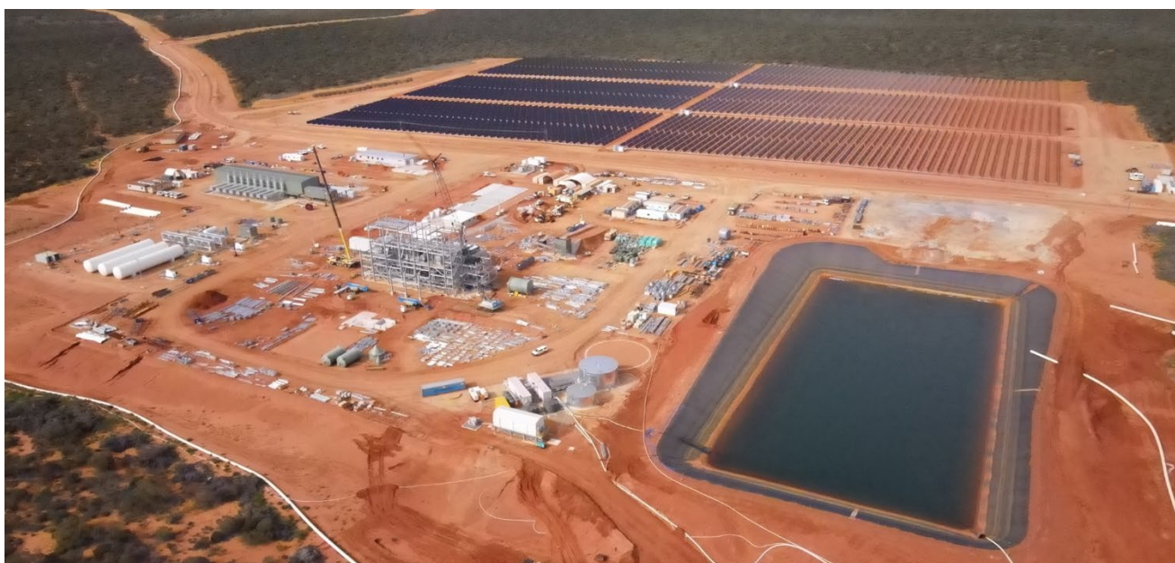
Figure 3 Construction of hybrid power station, MSP and supporting infrastructure advancing strongly in parallel with WCP
