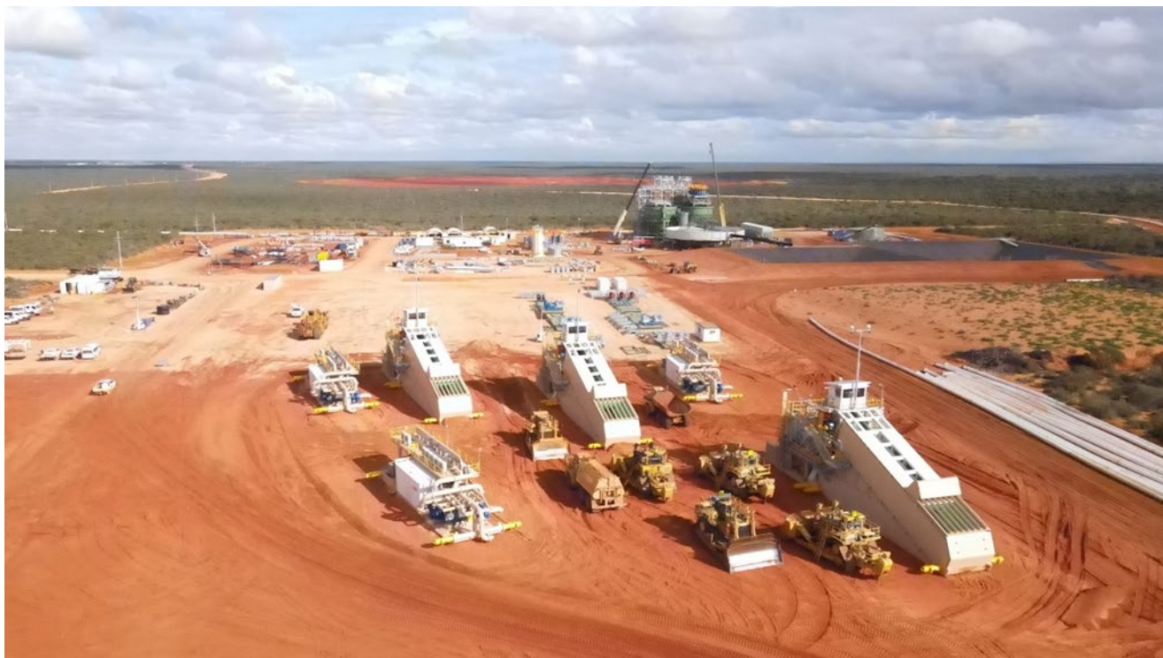
Figure 2 Development of Coburn's open pit mine has commenced. Dozer Mining Units ready to be moved into position
