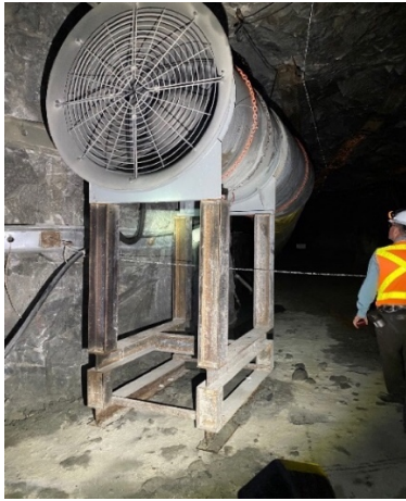
Photo 1 – Underground secondary fan
