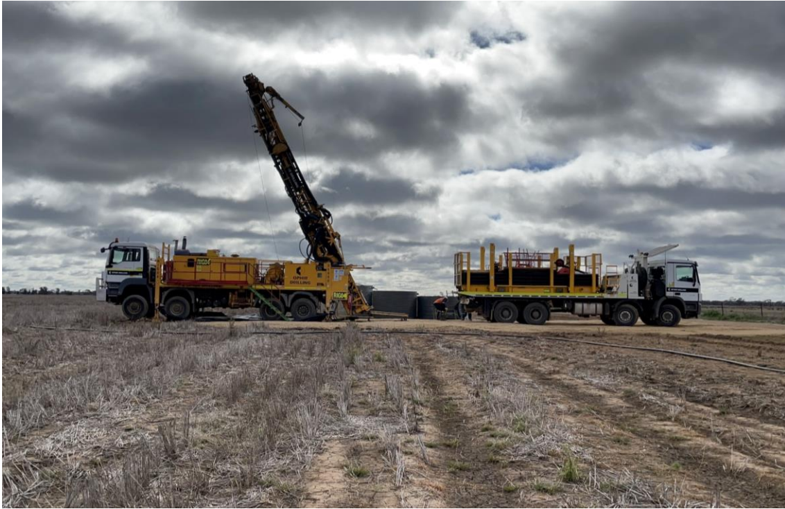
Figure 1. Diamond drill rig set-up at the site of the first drill hole (22MYDD414) at the Corvette Prospect.
