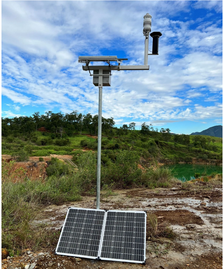
Figure 8: Sensors installed at the Mt Chalmers mine site.
