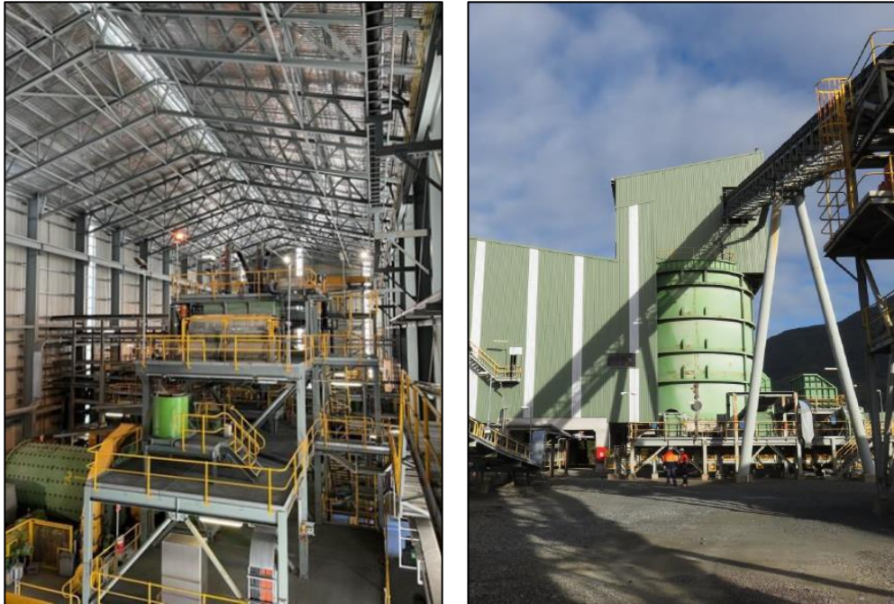
Figure 12: Plant infrastructure – grinding and flotation circuits (left); crusher house and fine ore bin (right) Source: Mallee Investor Presentation June 2022
