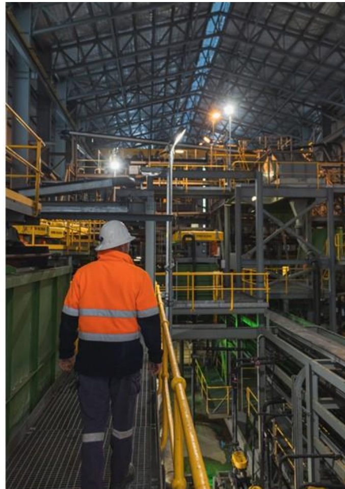
Grinding and Flotation Circuits
