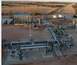
Gas Terminal DBNGP pipeline 4km from BSS
