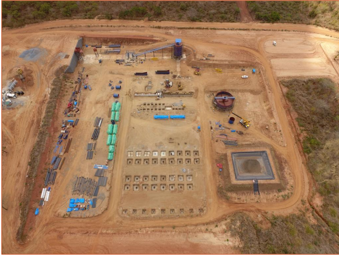
Figure 1: Mid-August 2022, oblique view from the south of the processing plant area. Development of foundations for the drying, screening and packaging building can be seen in the foreground with equipment delivered to site on the laydown area or being assembled and erected.
