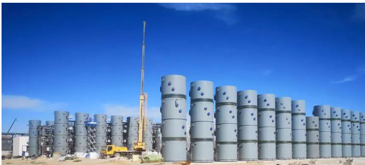
Figure 1: Zangge Lithium Plant supplied by Sunresin now in production. Plant constructed in 2018.
