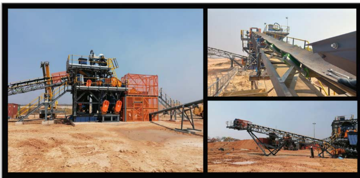
Lulo kimberlite bulk sample plant
