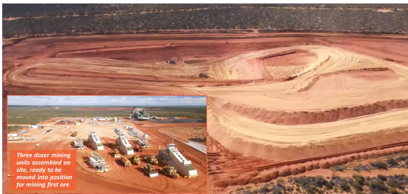
Figure 3 Development of Coburn’s open pit mine has commenced. Dozer Mining Units ready to be moved into position
