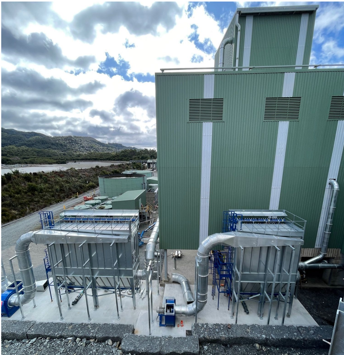
Figure 8: Dust Extraction System at the Crusher House
