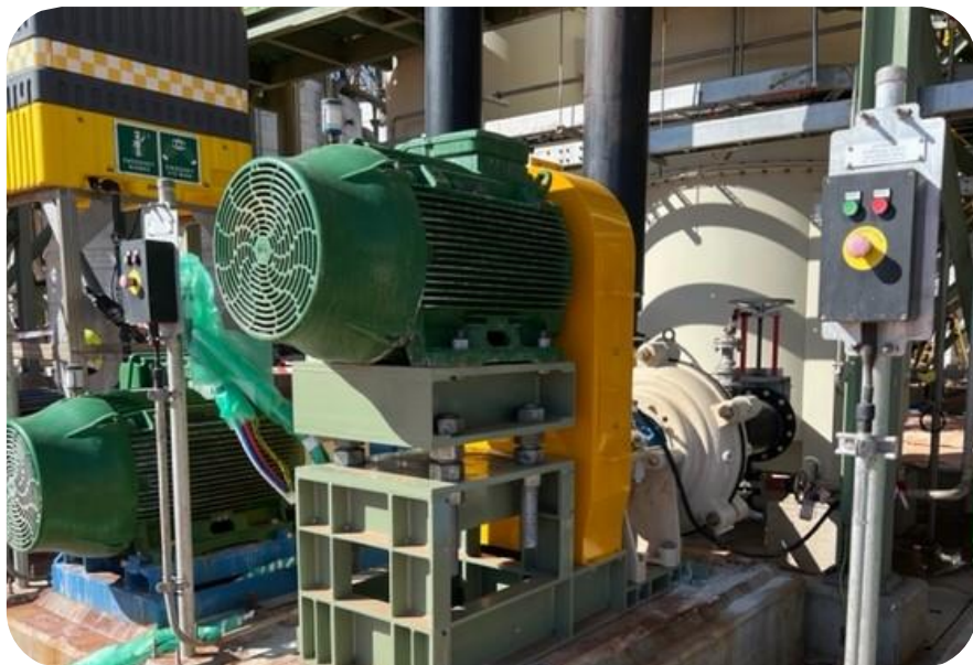
Flotation feed pump upgrade
