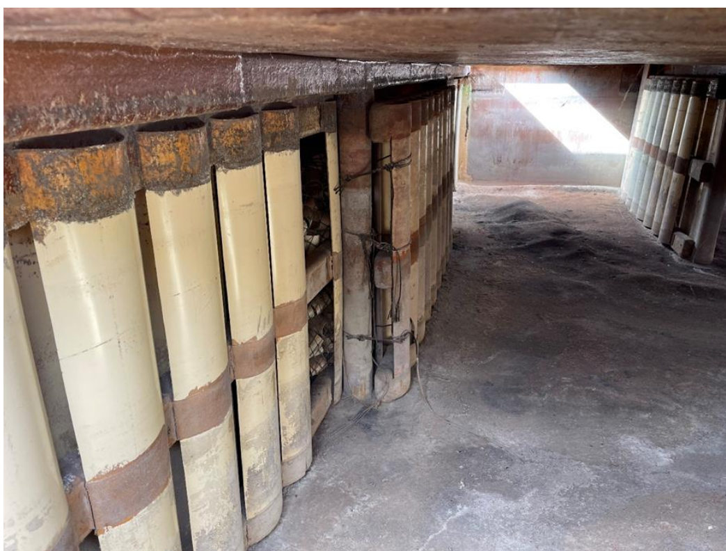
Image 1 / SX Mixer Settler cleanout lower level
