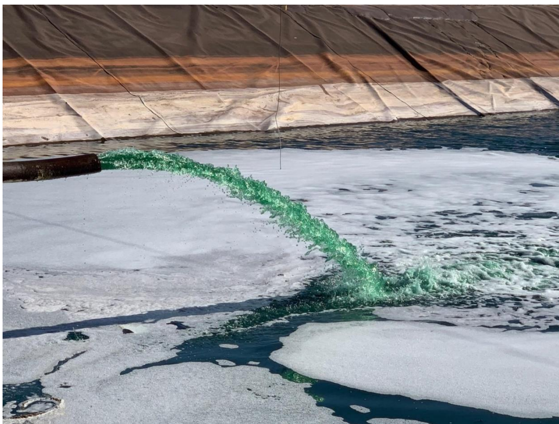
Image 8 / Copper rich solution being pumped to PLS pond for future solution inventory
