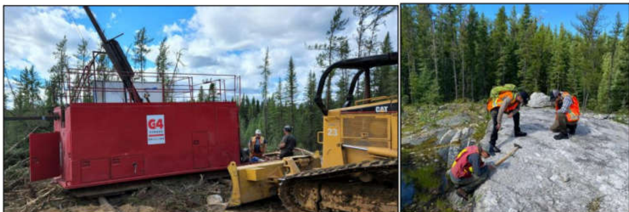
Figure 11 - Drill Rig preparation and LCT pegmatite outcrop at the Root Lithium Project
