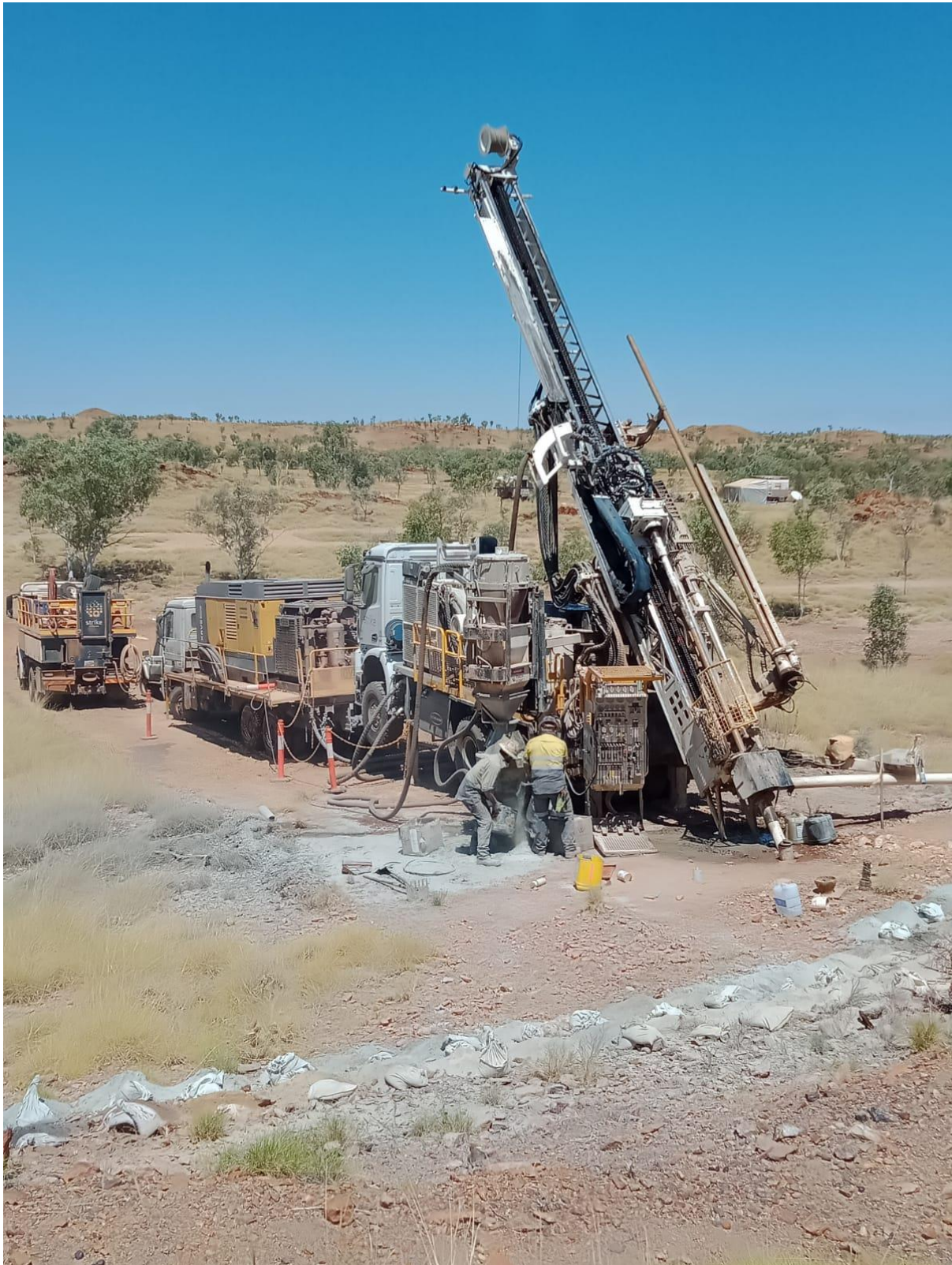
Figure 5: Drill rig in operation at the Horry Copper and Gold Project, Kimberley Region of Western Australia
