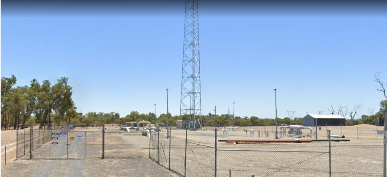
Image 1: DBNGP connection point located 0.3km from the Project
