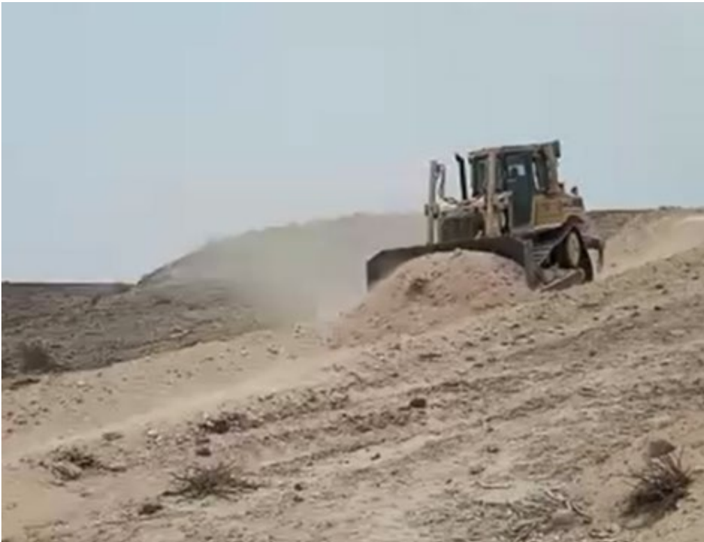
Figure 1: Dozer, operated by sub-contractor T-Angola, repairing a sandy section of access track.
