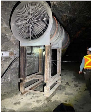
Underground secondary fan
