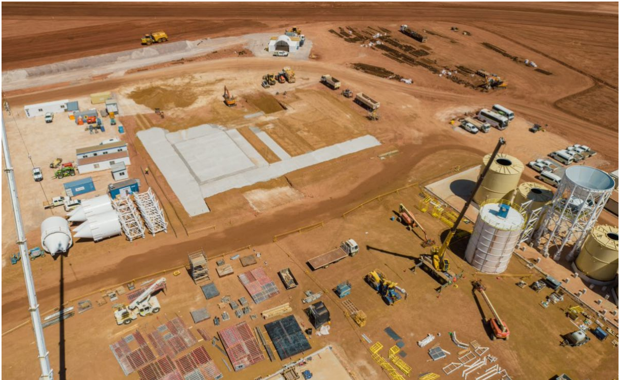
Concentrate Building Detailed earthworks and foundations complete and blinding in Progress, bolted soda ash silo nearing completion to right.
