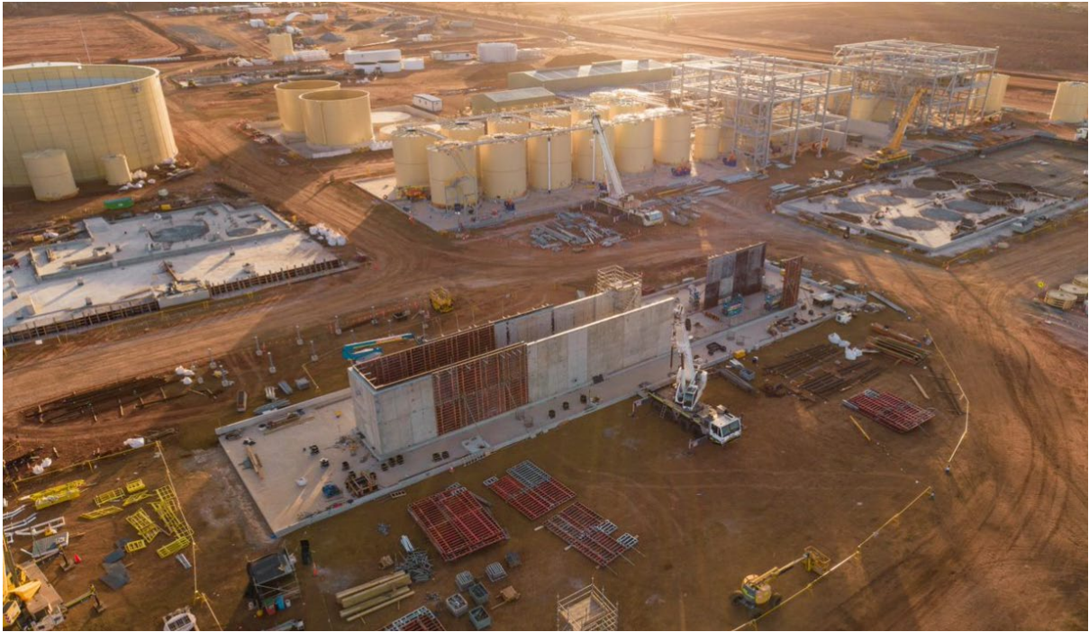
MgO Neutralisation tanks in foreground, tank farm and filter building in background
