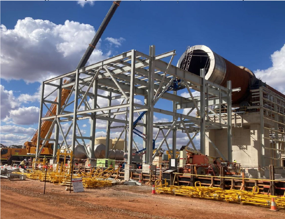
Feed Hood lower structure in place in preparation for kiln refractory installation
