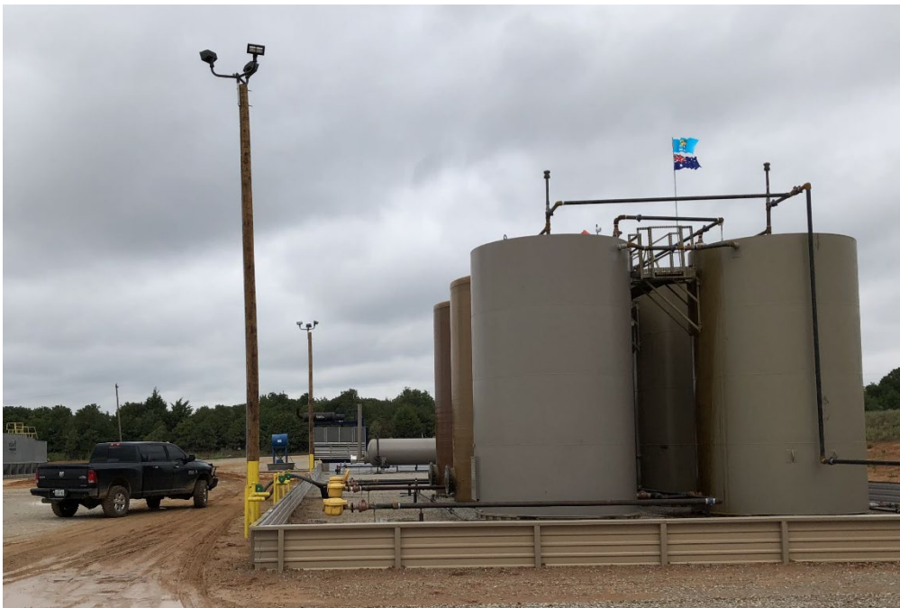
Figure 1. Flames Well Production Facilities in Carter County, Oklahoma
