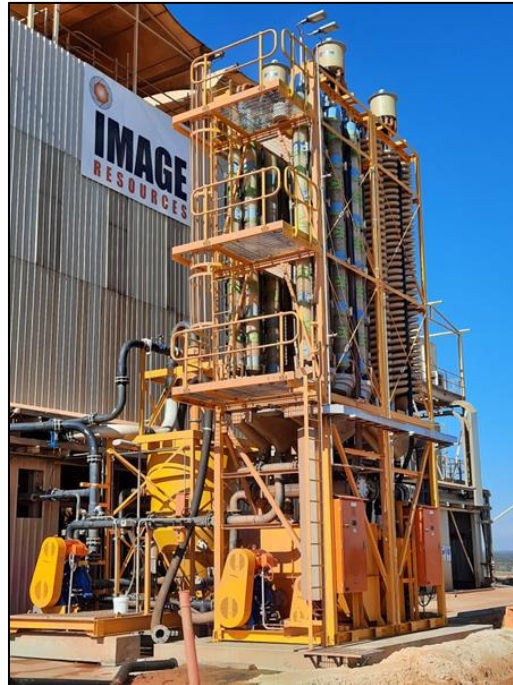
Photo 1: CT1 Demonstration Plant
