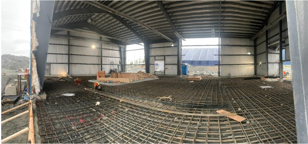
Figure 2: Conversion of crusher building into maintenance workshop (preparation for pouring of concrete pad and access doors established)
