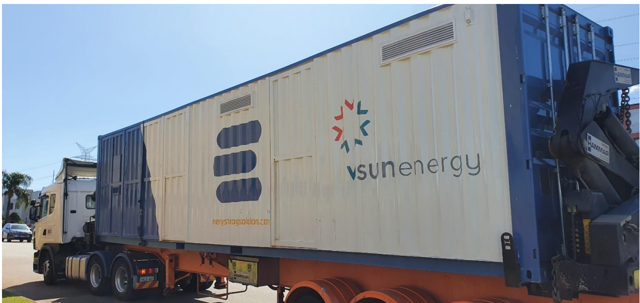
Figure 5 IGO SPS VRFB en route to CDI Electrics for FAT
