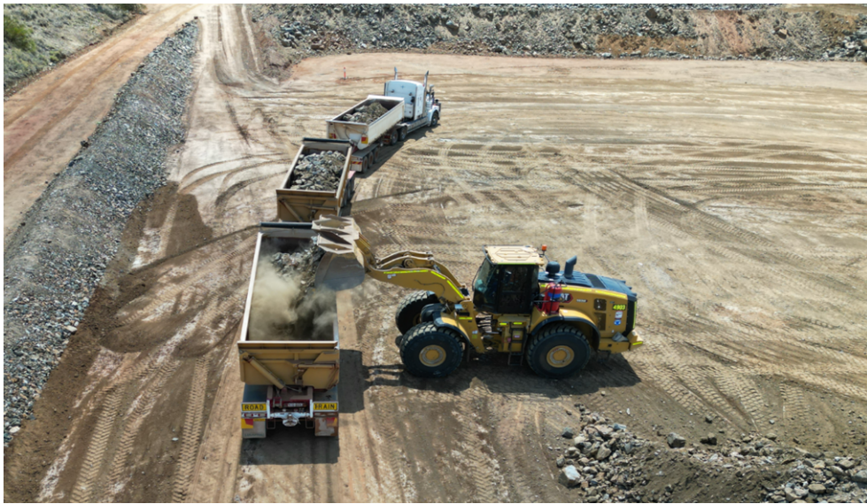
Image 2 - First materials being loaded - Main ROM at top of image ready for transport and processing currently containing a combined 72,545 tonnes
