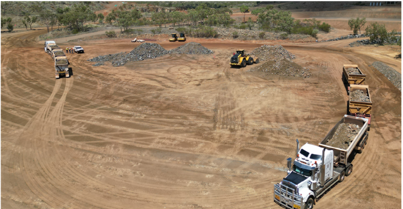
Image 1 - The Initial two triple road trains being loaded with material from the Comstock pit for delivery to the GAM Plant for processing and first gold production
