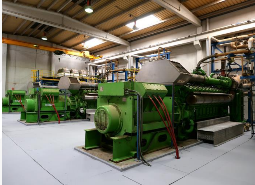
The El Romeral Gas to Power facility
