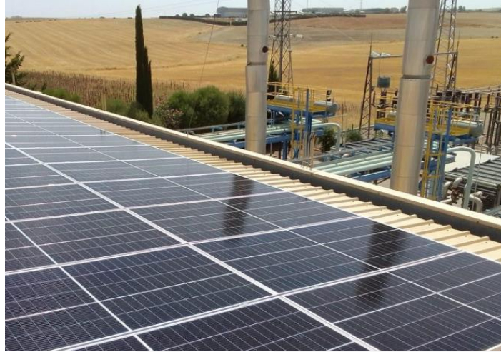
Part of the solar panel array installed on the rooftop of the El Romeral power facility, Spain.
