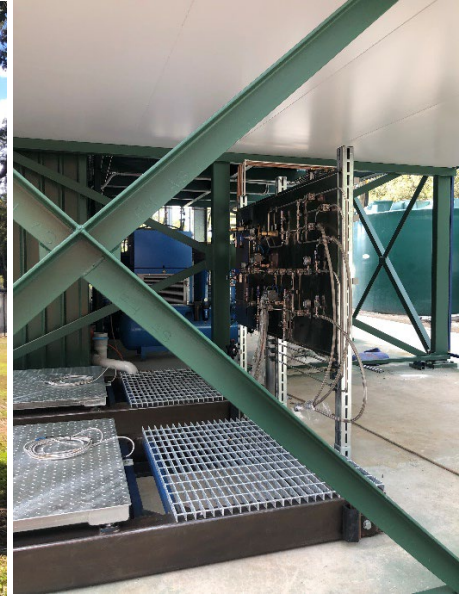
Hydrochloric acid gas manifold
