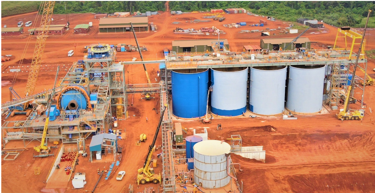
Figure 2: CIL tanks at Abujar are functionally complete
