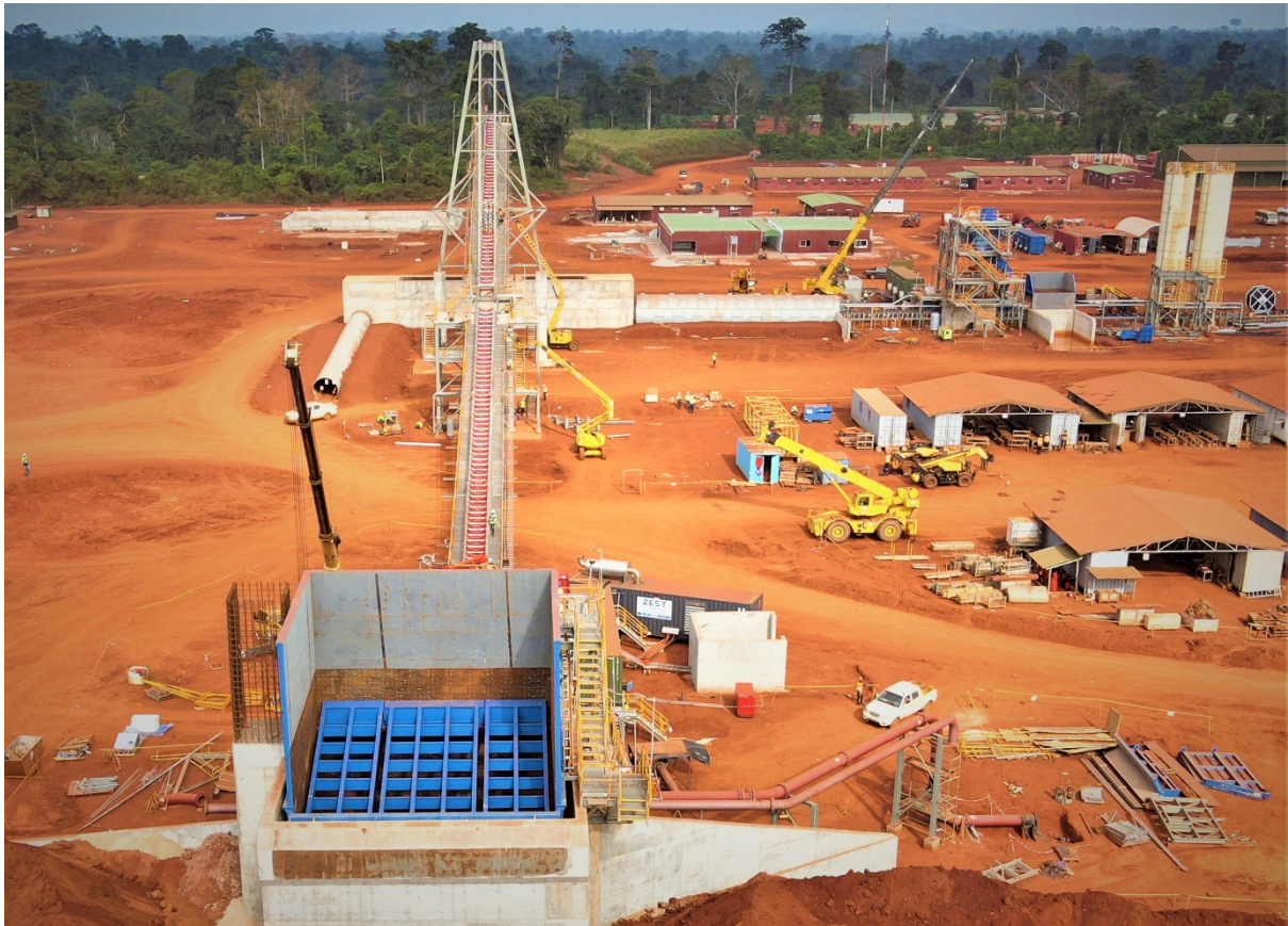
Figure 5: CV-01 and reclaim
