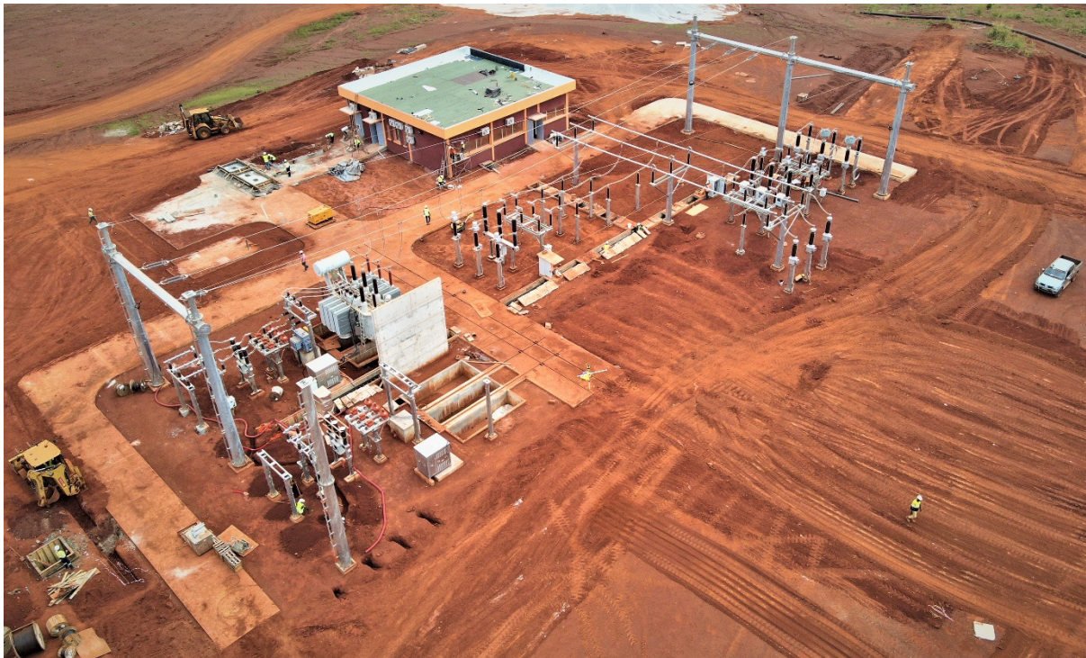
Figure 9: Abujar 90 KV substation
