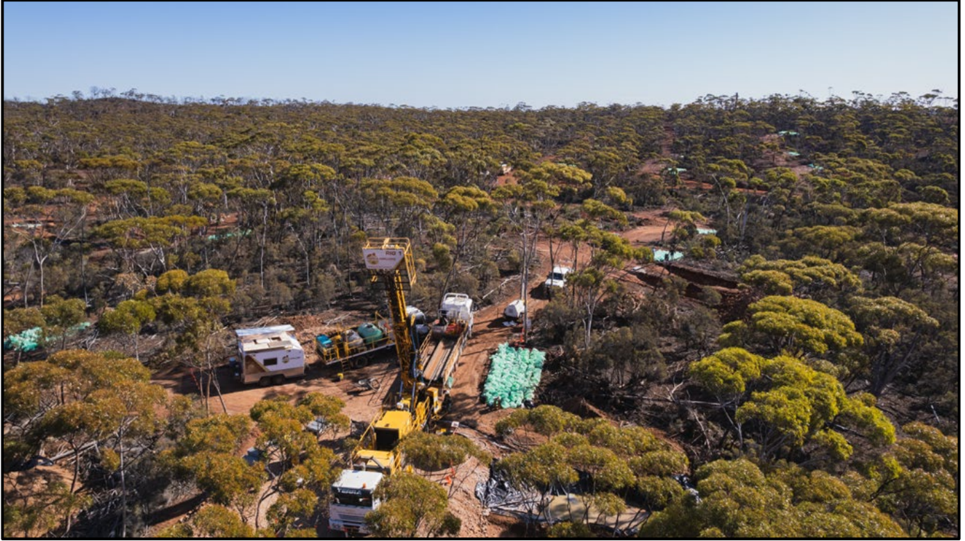
Figure 1 – Diamond core drilling on site at Callisto with completed drill sites in the background. Drill pads and track clearing are designed to minimise the environmental footprint of drilling. All diamond core holes to date have been pre-collared with RC drilling which saves time and money.
