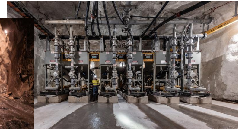
8 Level Underground Pump Station
