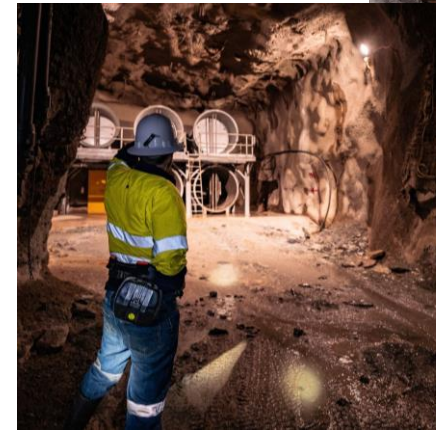
7 level Underground main fan installation
