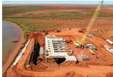
SEAWATER INTAKE STATION
