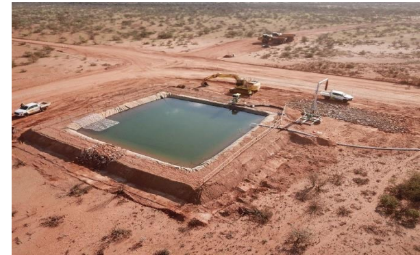
Figure 4. Turkeys nest for construction water
