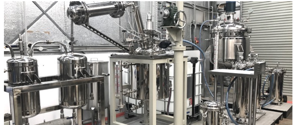
New iBC® Pilot Plant, installed at Victoria University, in Victoria, Australia.
