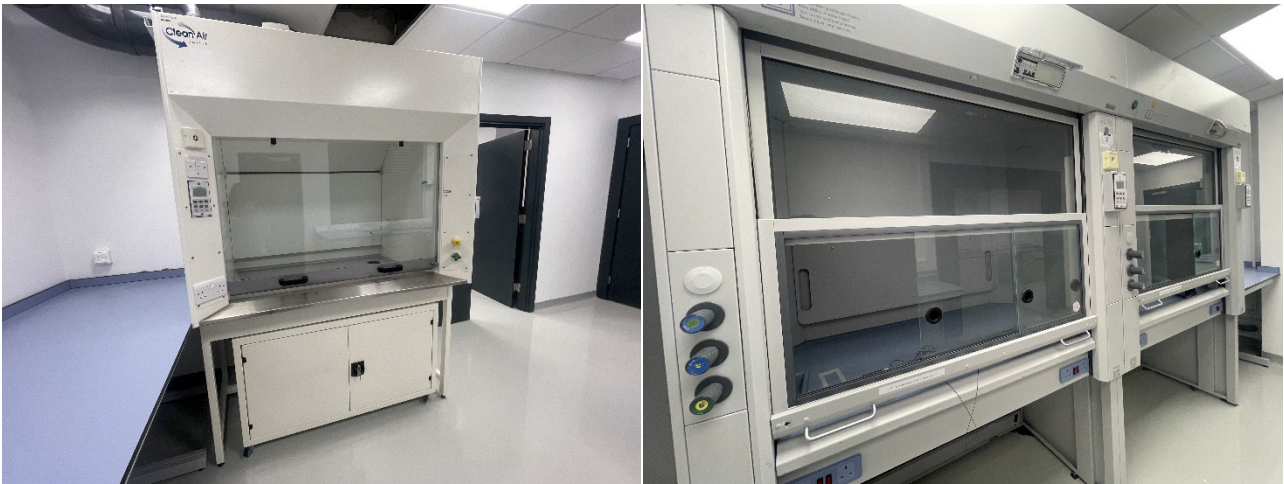
Figure 6: Benches and fume cupboards installed across several wet hydrometallurgical labs.
