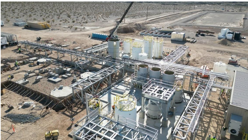
Figure 1 – Construction of the Fort Cady Complex in Southern California (Dated December 19 th , 2022)
