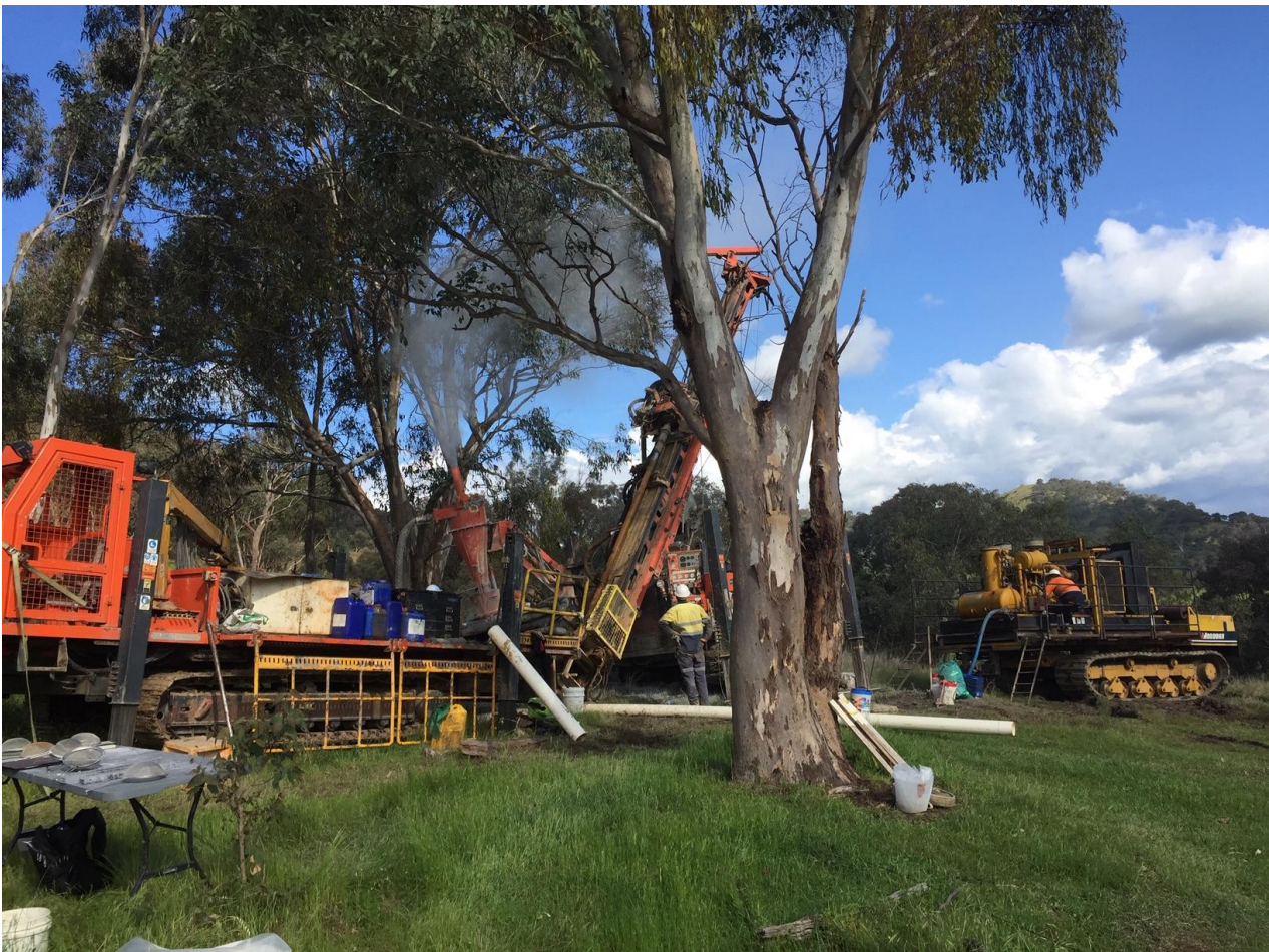
Figure 2: Drill Hole 3DGIB007 being drilled 120m North that intersected several high grade intersections. However, located behind the Compressor to the right of this photograph is an additional group of surface workings that have yet to be drilled
