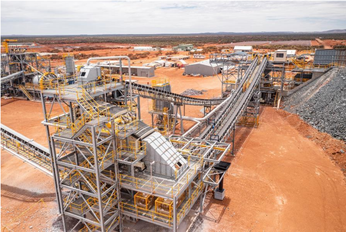
Figure 4 – Processing plant crushing section commissioned in December quarter (Photo – 20 January 2023).
