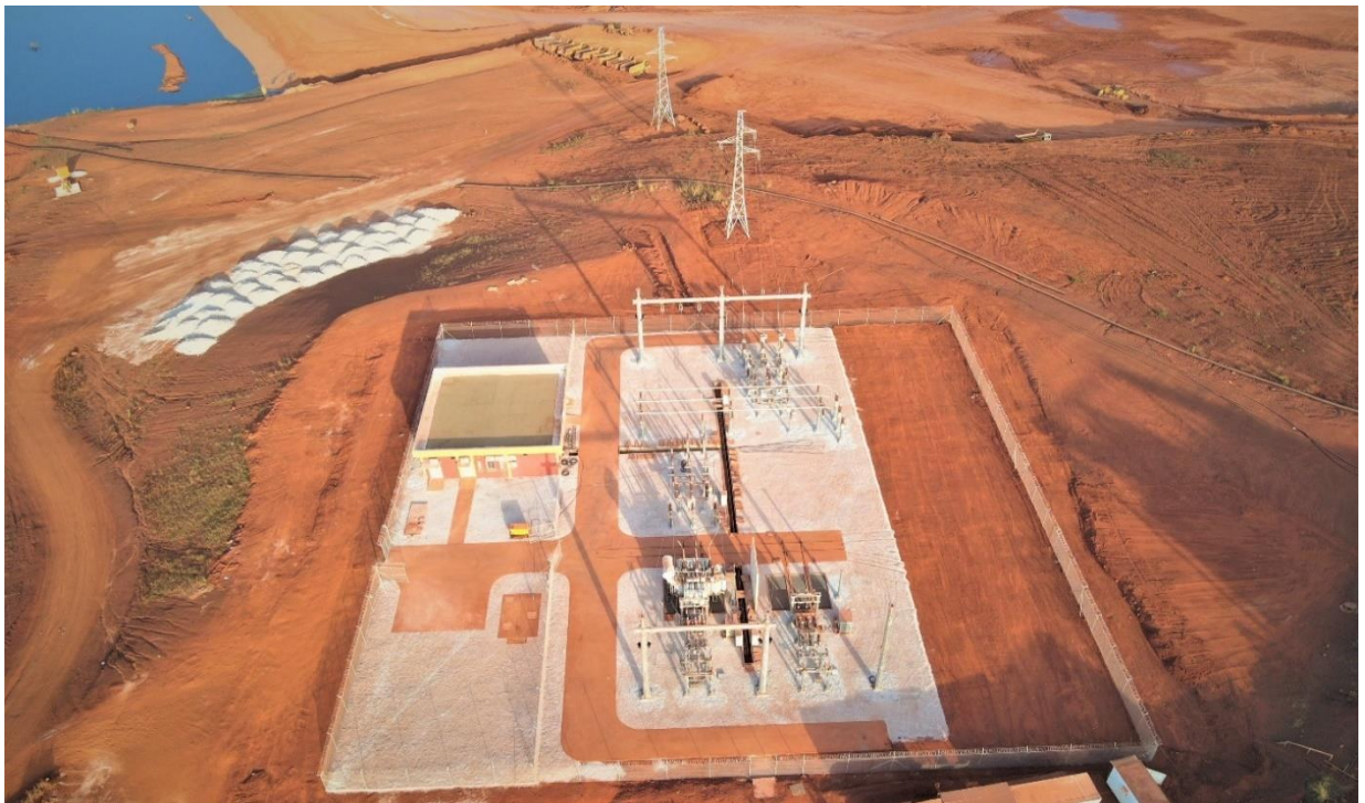
Figure 8: Abujar 90kV substation
