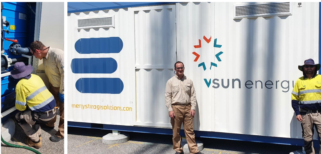
Figure 6 - E22's engineer Veselin Miroslavov and VSUN Energy's Principal Electrician Lee Bourke pictured alongside the VRFB for IGO
